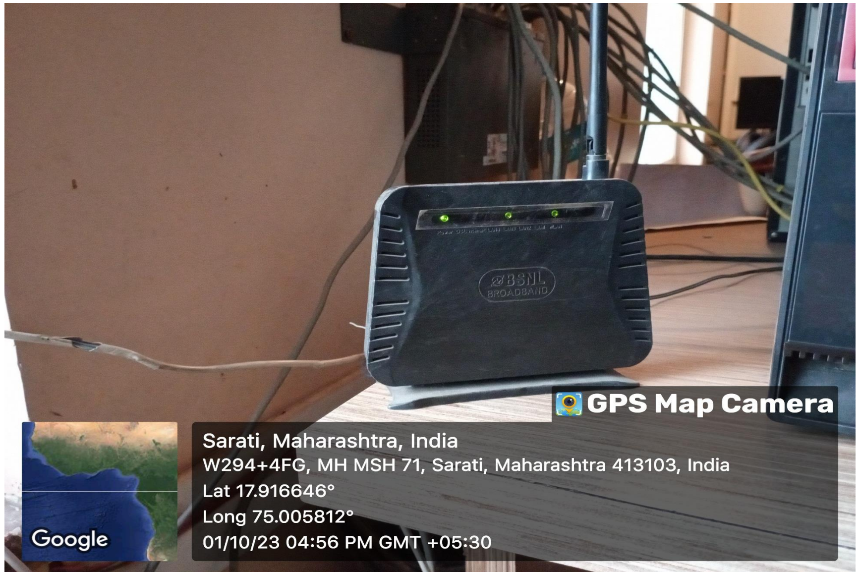
Wi- Fi Router 1
